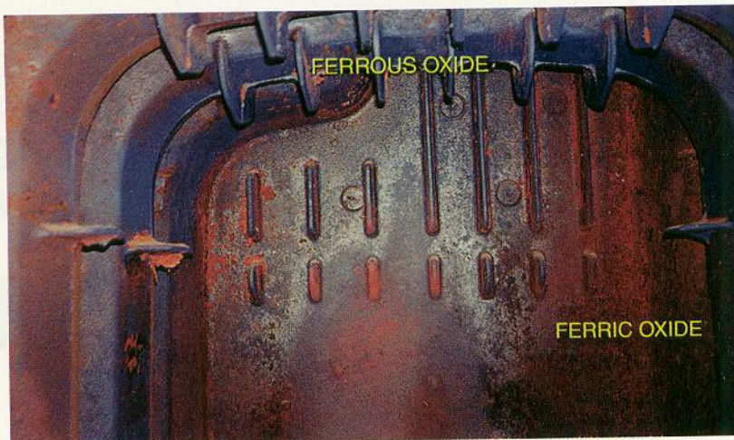
Discoloration of cast iron boiler sections indicates overheating did occur.
